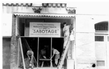
New Theatre Exterior Under Construction 1943 exhibition print from original gelatin silver photograph 29.7 x 42 cm Arts Centre Melbourne Performing Arts Collection Gift of Dr Angela O'Brien 2001
